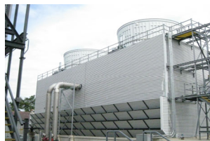
Example of a cooling tower at the University of Illinois - Urbana Champaign
