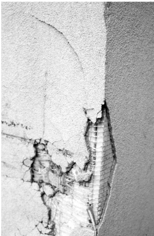
Figure 5. This photo of easily damaged EIFS reveals the layers of construction. Source: Fred Schlipf.
