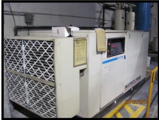
Photo 5: HP Air Compressor
