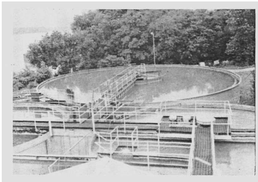
Figure 6. Two mixers in foreground with clarifier in background
