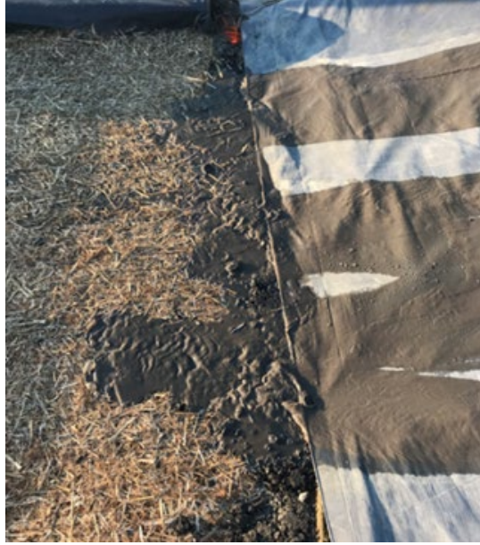
A. Water passed underneath the blanket
