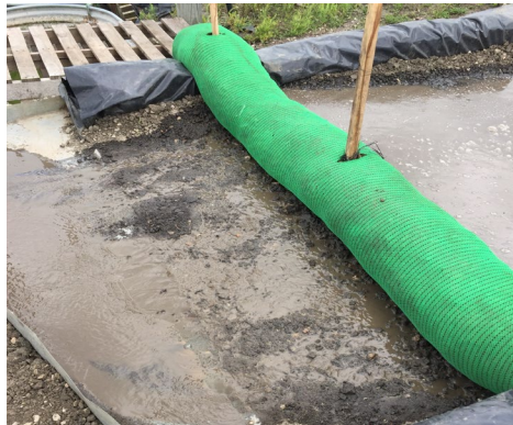
A. Flow draining out of the bottom of Filtrexx Siltsoxx
