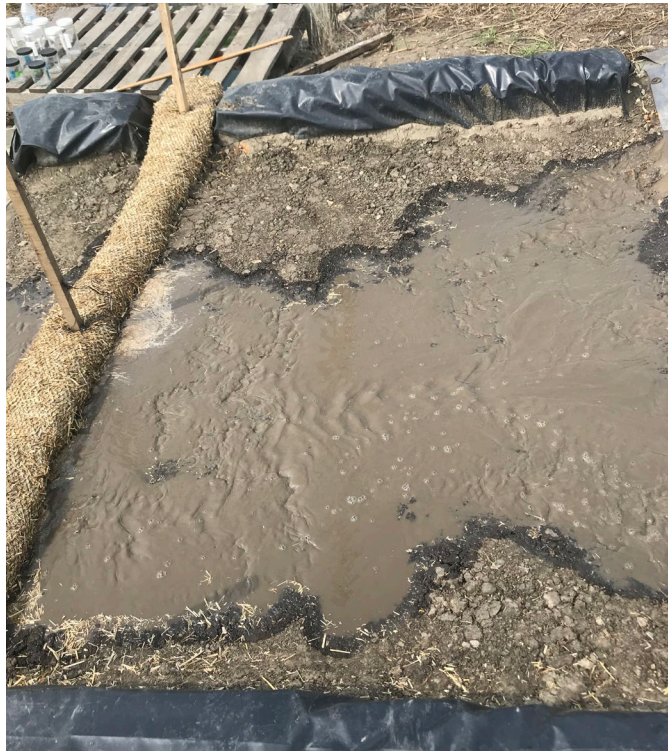
Figure 34. Photo. Almost no ponding upstream.
