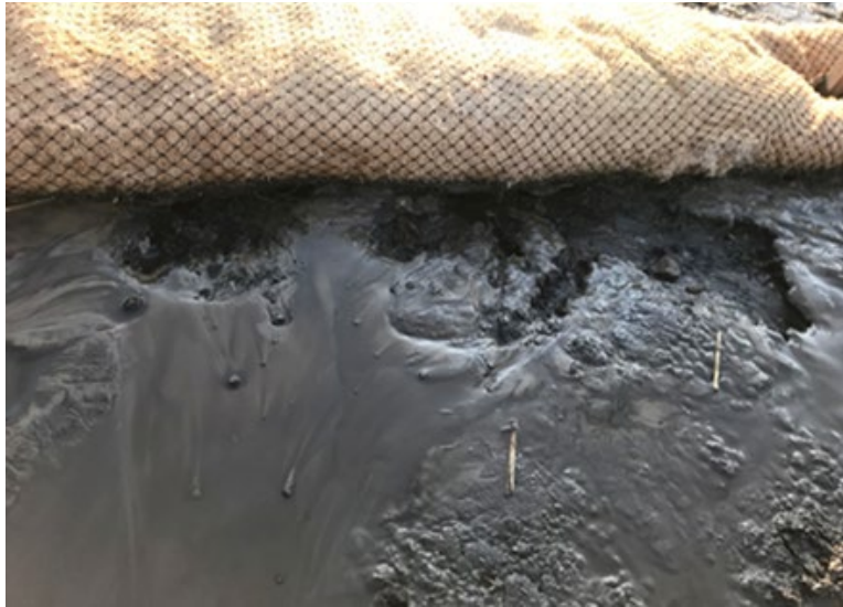
A. Undercutting upstream
