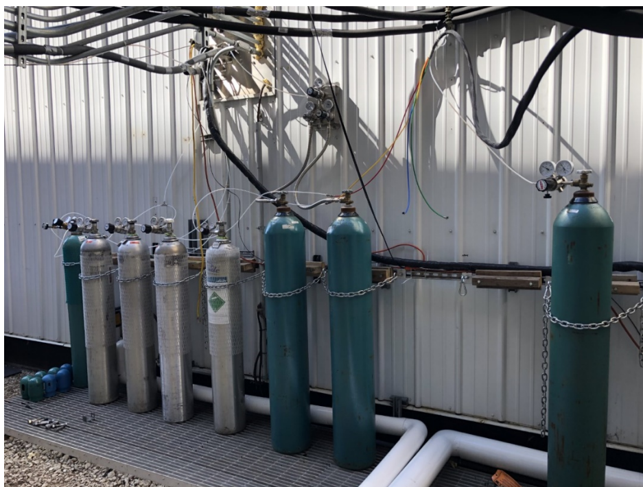
Figure 2.13. Calibration gas cylinders next to the analytical trailer. Each gas was regulated and passed through a bulkhead that went to the SAS or remained outside to go to the FTIR system.
