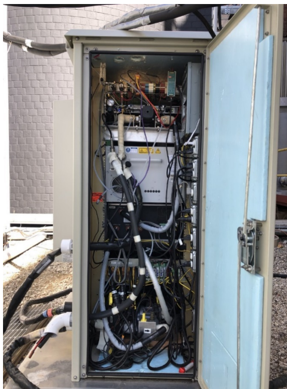
Figure 2.10. Interior of the rear-side of the FTIR cabinet.
