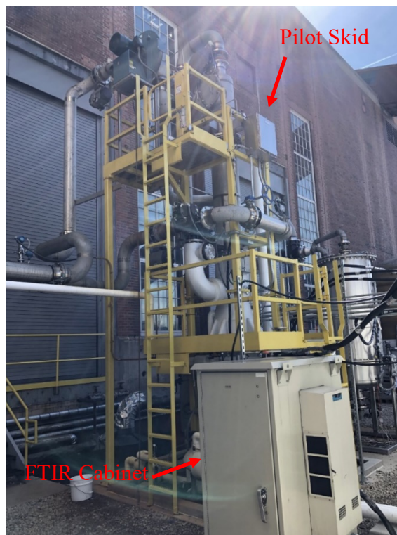
Figure 2.5. South facing view of the pilot skid and Fourier Transform Infrared Spectroscopy (FTIR) cabinet at Abbott Power Plant.
