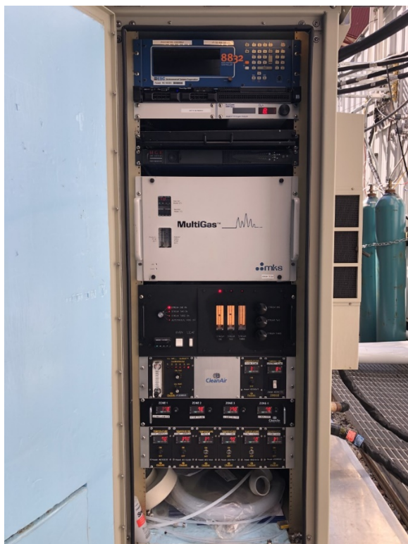
Figure 2.9. Interior of the front-side of the FTIR cabinet. From top to bottom, the components are: datalogger, O 2 analyzer, control laptop, FTIR analyzer, flow control box and temperature controllers.
