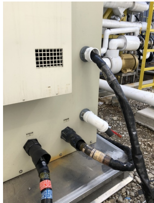
Figure 2.8. Heated sample lines going to the FTIR cabinet. From bottom left to upper right corner, the sample lines are return, supply, bypass and flow to the SAS.
