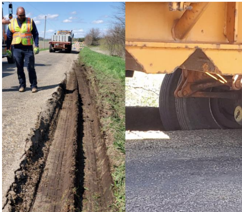
Figure 2.20. Damage of the road due to heavy axle loads during the proof load test
