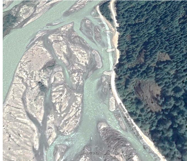
Figure 22: Erosion control measures along the eastern side of the Braided Reach to protect the Squamish Valley Forest Road from Google Earth, 2023
