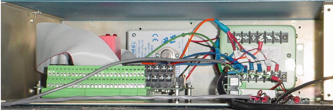
Figure 5.19 - The actuator optical isolation box
