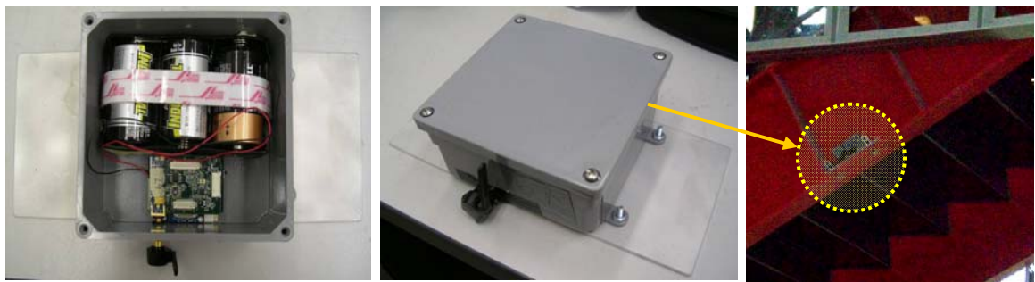
Figure 7.86 Siebel Center staircase (top) with sensor nodes installed (bottom).
