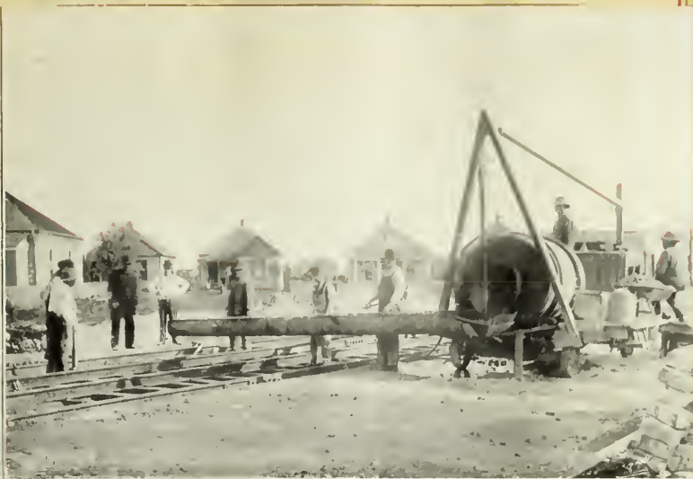
Illustration showing the Eclipse Mixer on Street Railway Work. The long trough is used to convey concrete over the tracks and is swung to one side for cars to pass.
