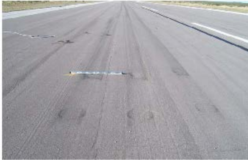
Figure C.1 Rutting in asphalt with tire imprints – Runway 22 touchdown area.
