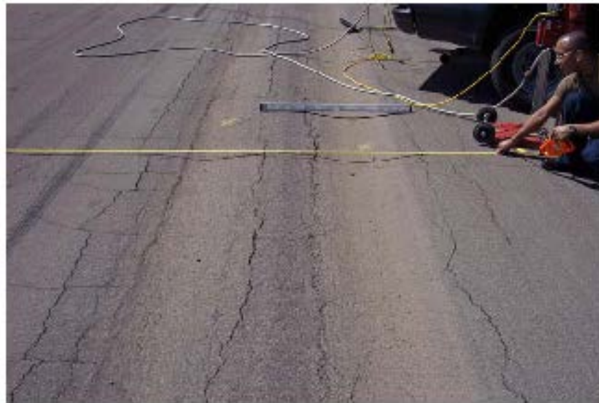
Figure C.2 Runway asphalt distresses include cracking and rutting.
